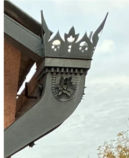
Down Spout on Building in Sloviansk
